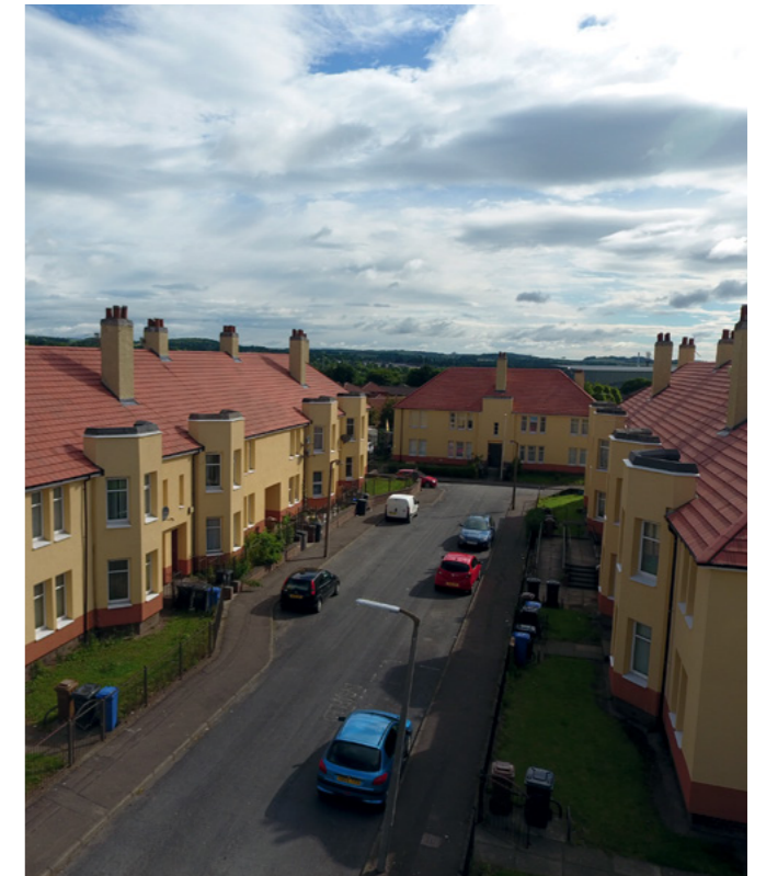
Dundee - Dundee Basic1 system consisting of 100mm Enhanced EPS. The alsecco system has been installed to over 2500 units across various locations. The ongoing project has not only improved the aesthetics but fundamentally the thermal efficiency of the existing building.
