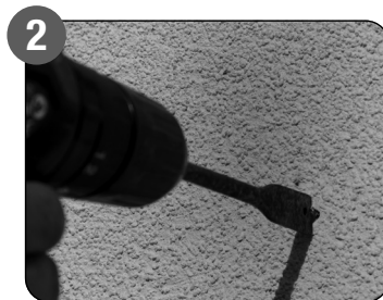
2 Mark position and drill pilot hole through the render at 300mm centres.
